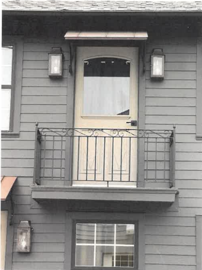
Photo 2 – Example Balcony Handrail & Appearance
